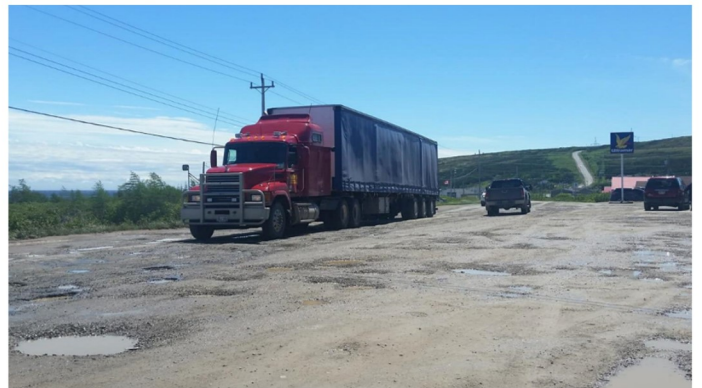
Figure 3: Potholes on highway 510 in Forteau NL, July 2017.
